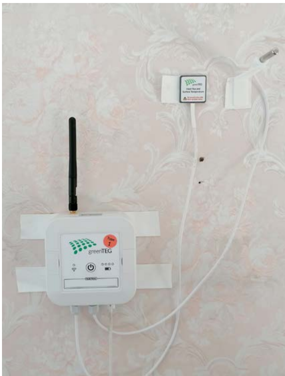
Figure 16: In-situ U-value measurement kit installed on the internal face of a wall (note that the presence of wallpapers may distort the reading)
