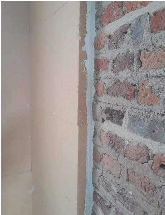
Figure 55: Build-up of lime mortar to level uneven surface prior to application of woodfibre board
