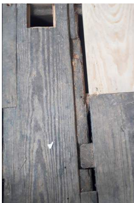
Figure 38: Care must be taken when lifting existing floorboards to conserve historic detailing like this biscuit joint
