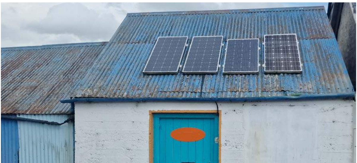
Figure 67: PV on the roof of an outbuilding
