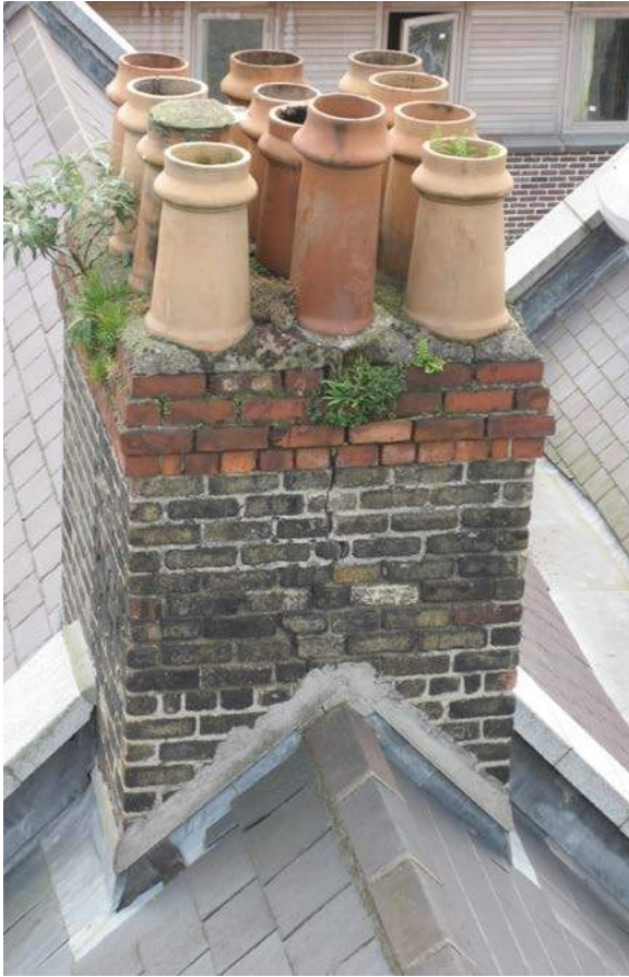
Figure 35: Traditional chimney stack requiring repair and maintenance
