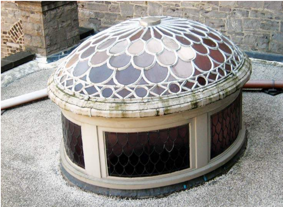
Figure 37: Historic skylights and lanterns, such as this fine example, should be well maintained but can be difficult to upgrade thermally. Consideration should be given to adding secondary glazing at ceiling level (Image from Advice Series: Energy Efficiency in Traditional Buildings , 2010)
