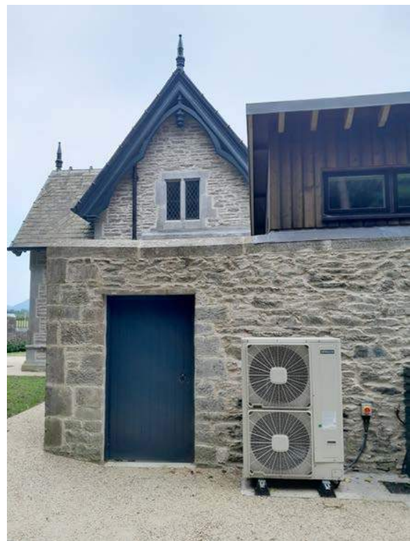
Figure 63: Air source heat pump
