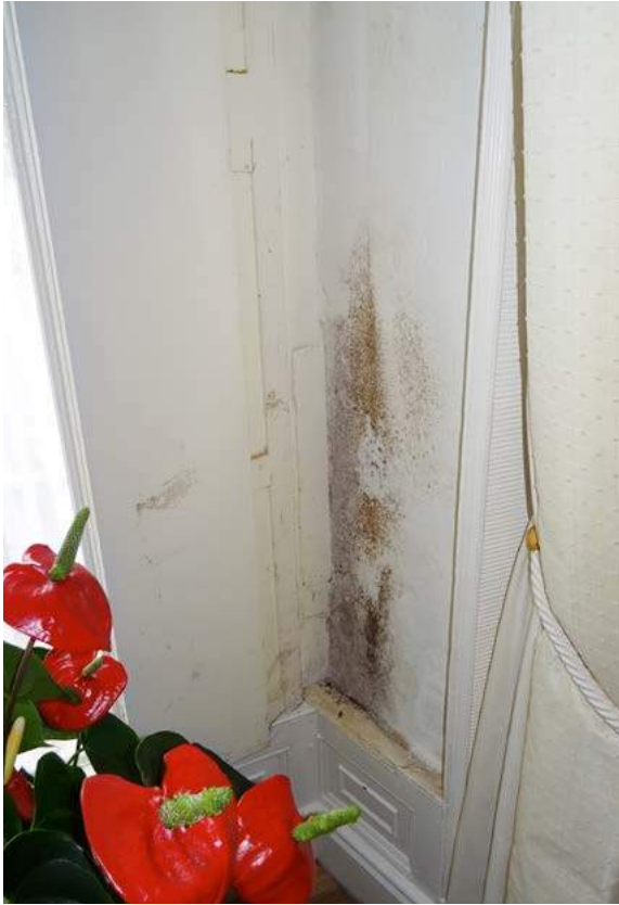
Figure 17: Mould growing behind shutters
