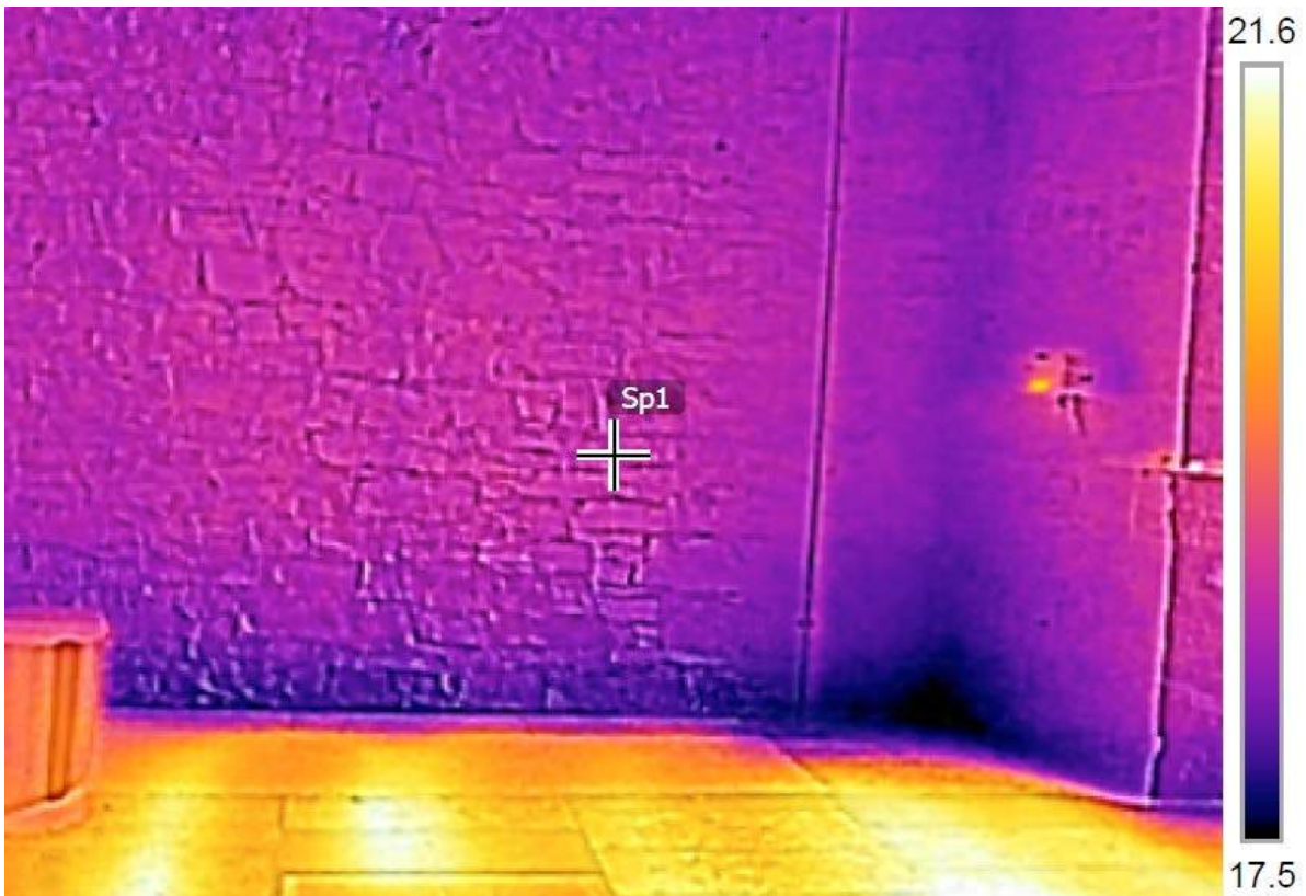
Figure 10: Thermal image showing additional heat flow at vertical and horizontal junctions with the abutting walls and floor. Note that the corner is the coldest point because it loses heat in three dimensions
