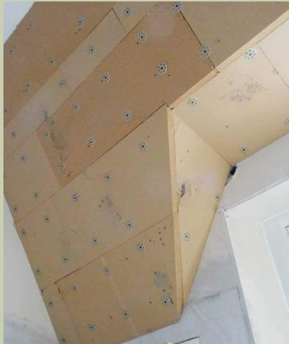
Figure 34: Wood-fibre insulation board fixed to the internal face of rafters. Thermal modelling may be required to ensure the minimum surface temperature is achieved in accordance with TGD L, Appendix D
